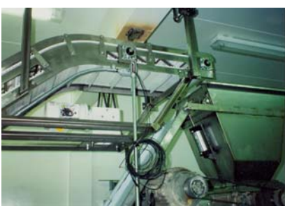
Scrap Conveyor standard discharge and metal detector discharge shut.
